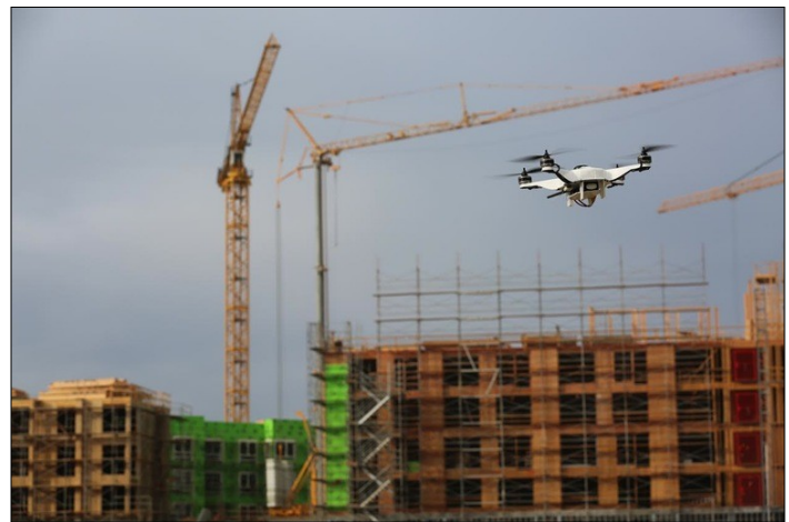
Project in Japan under observation with use of drone (Smart Construction initiative)
