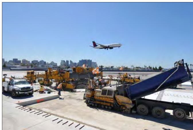
Flatiron Construction of the concrete apron construction adjacent to the new Landmark Aviation facility (Fleet Base Operator) at San Diego Int'l Airport
